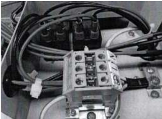
Terminal block connected
